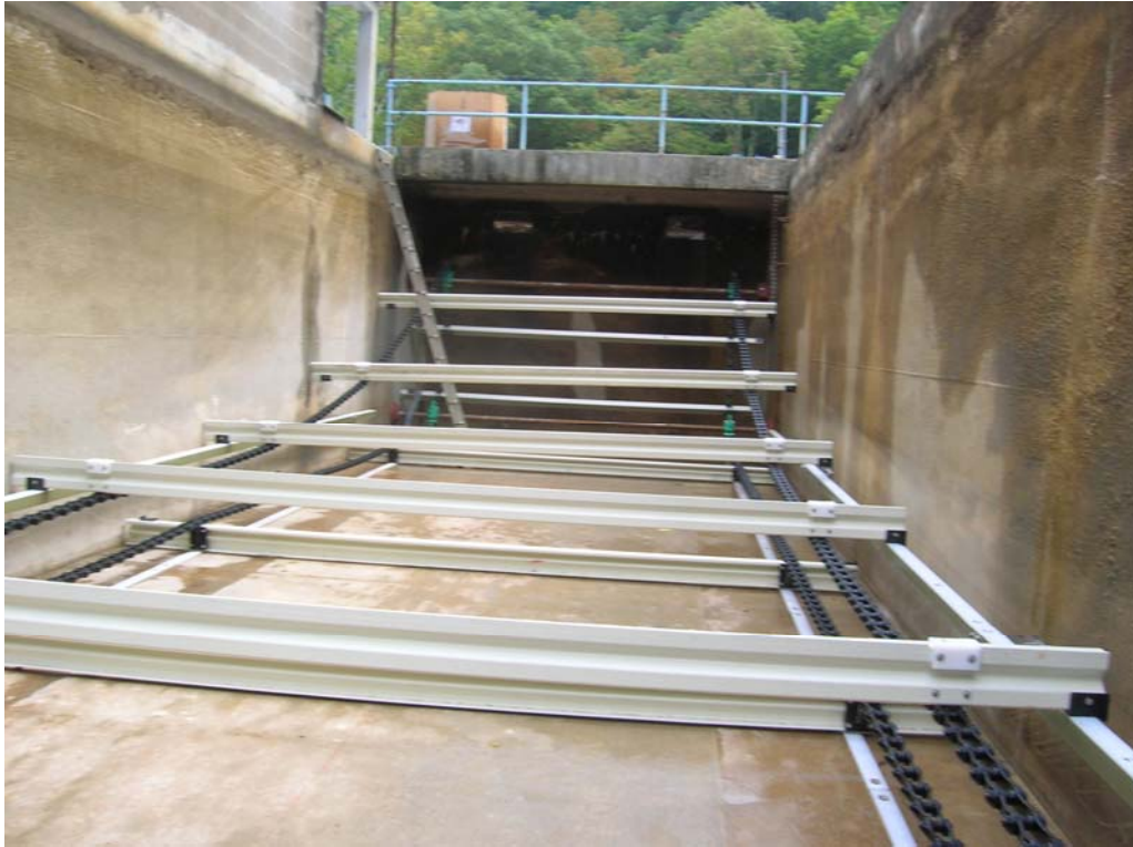
Chain & Flight Sludge Collector Installed in Settling Basin
