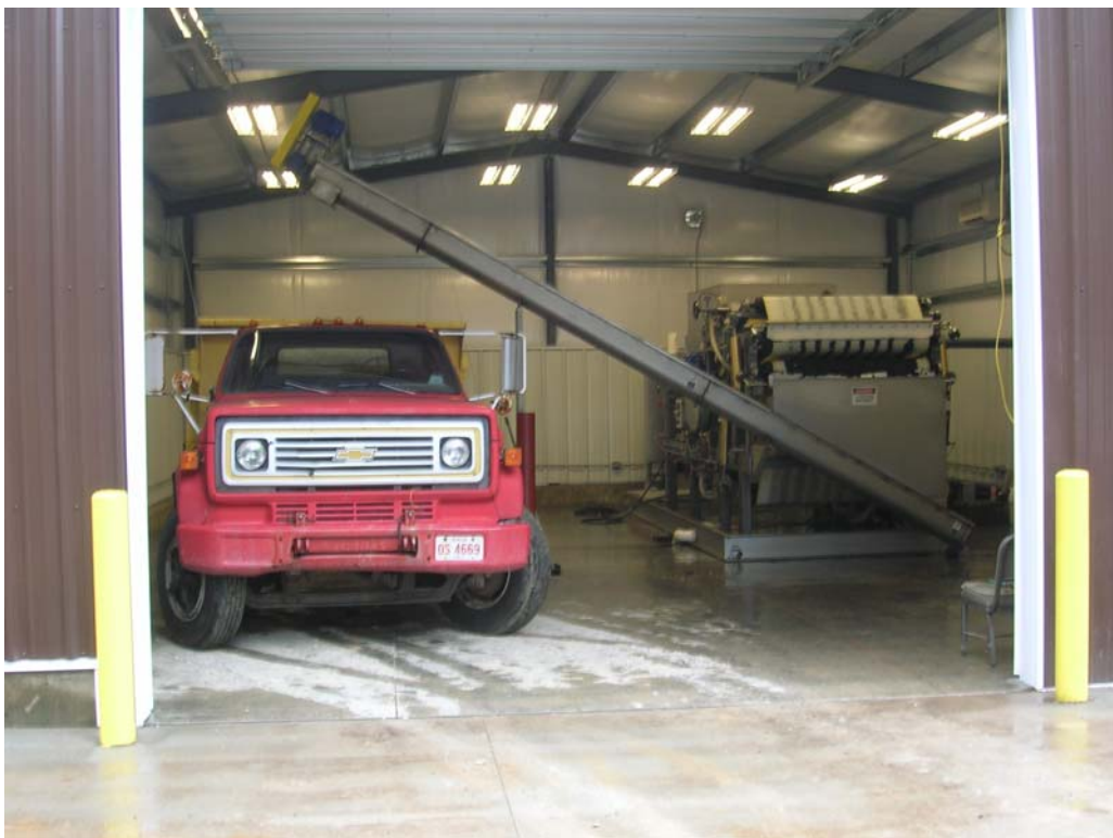
Belt Filter Press in operation in April 2009
