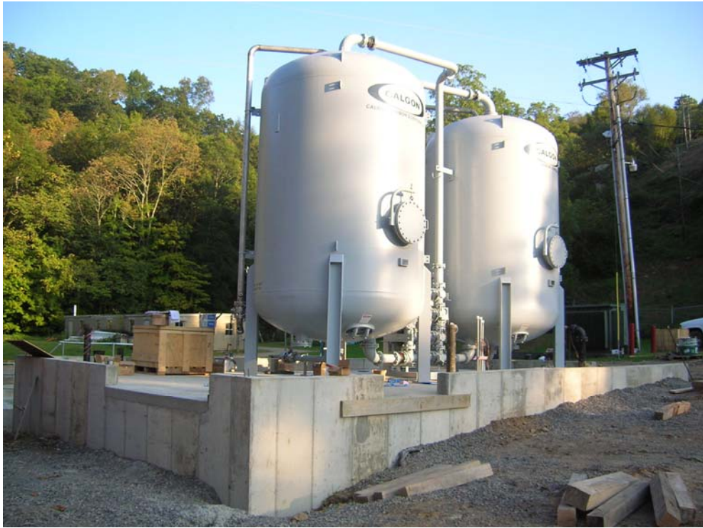
GAC Filter Vessels Installed on Foundation
